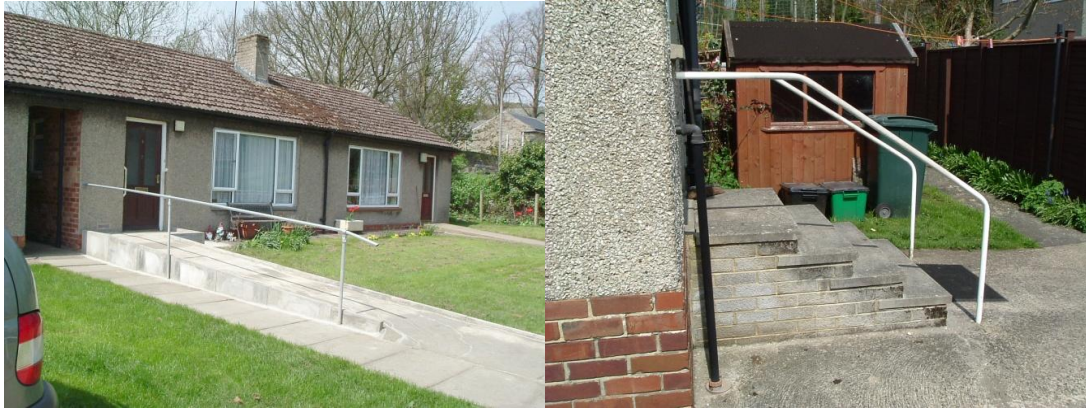
Figure 14 Social Housing in “Upperdale”: With ramp conversion (left); original front door steps (right)
