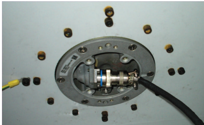
Figure 86 - pump installed in CARAD Times rig
