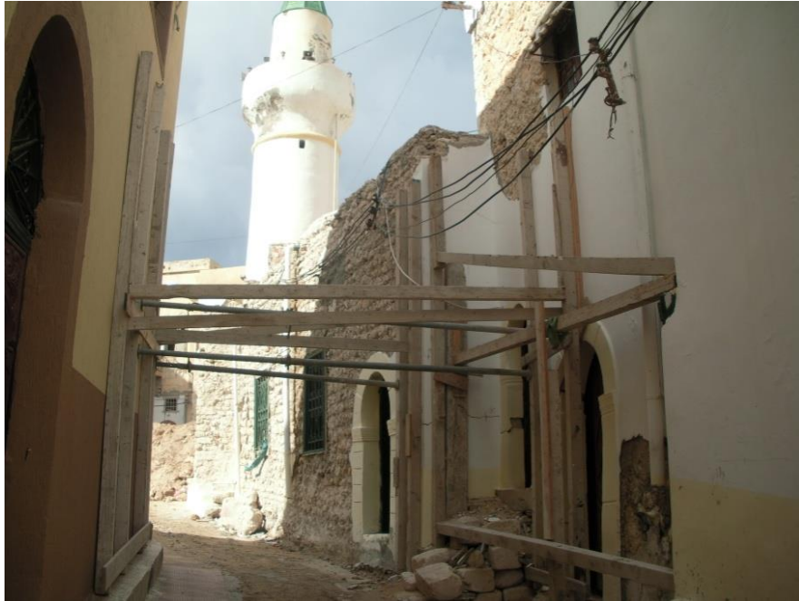
Figure 6.10: Jama al-Mushat Tripoli, showing the risk of falling during work (the author, 2010)
