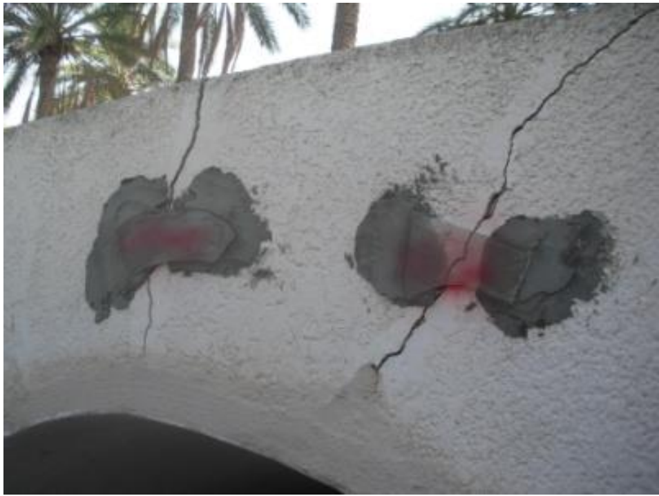
Figure 6.11: Monitoring the wall cracks in the Islamic museum project (the author, 2010)
