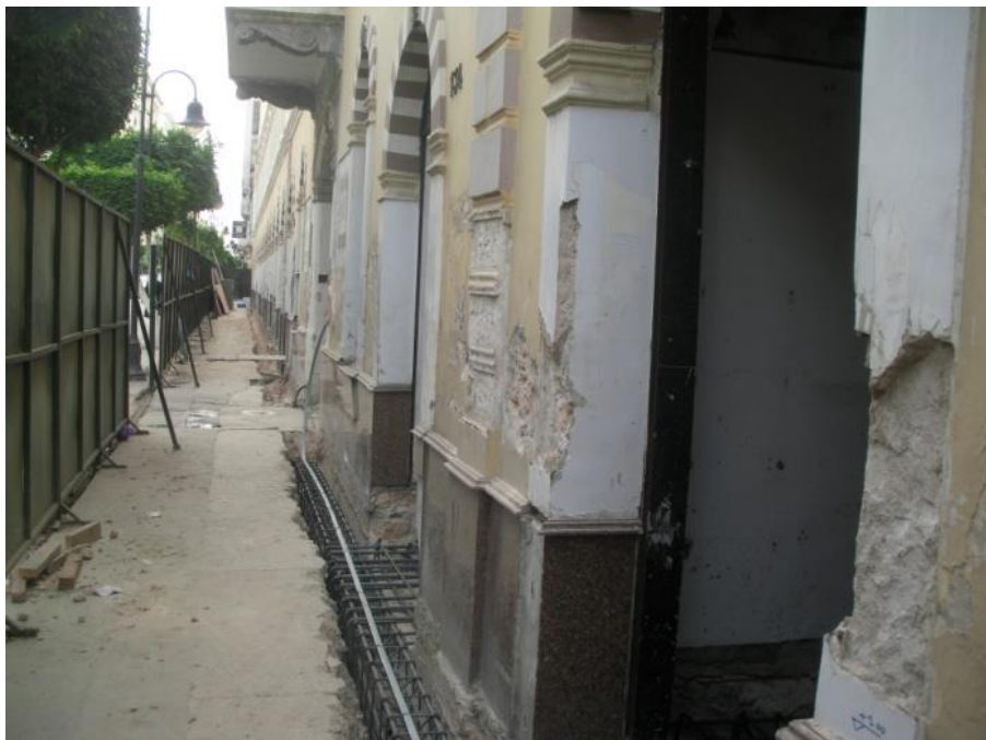
Figure 6.12: Supporting the foundations of the arts and crafts school, Tripoli (the author, 2010)
