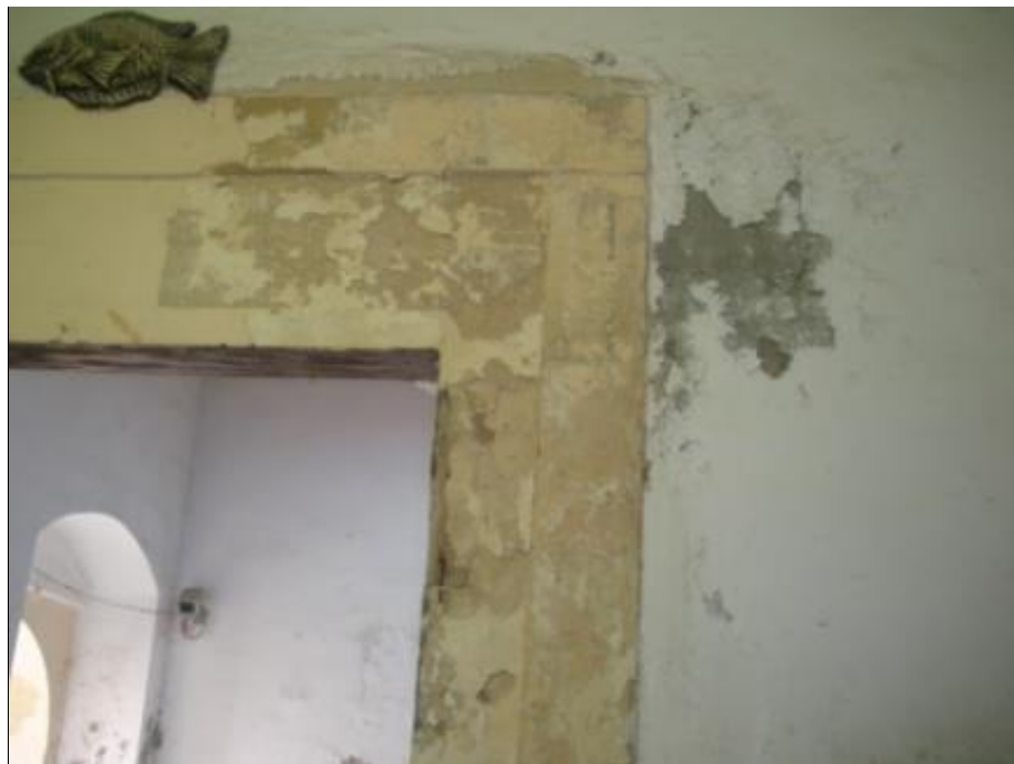
Figure 6.4: Humidity in walls, the former British consulate in Tripoli (the author, 2010)
