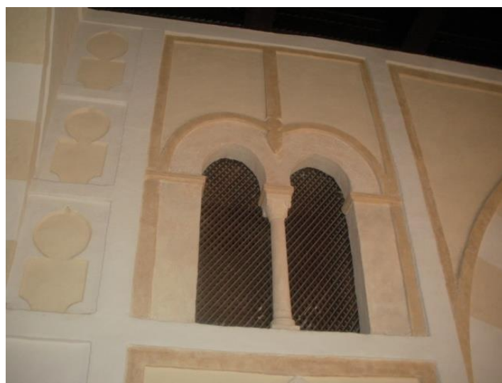
Figure 6.9: Paint grades that were adopted in the Islamic museum project, Tripoli (the author, 2010)
