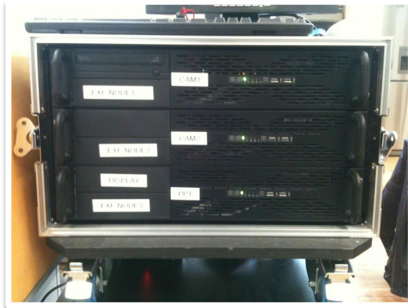
Figure 31 Flumotion Venue Nodes (Rack 1): Three rack machines – two for camera capture and encoding, one for VGA capture and encoding.
