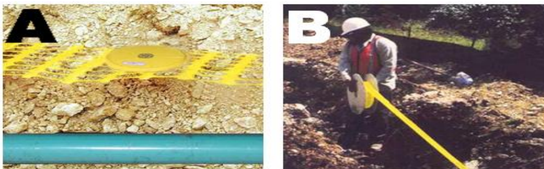
Figure 4-4: Pipeline installation activities: (A) A typical fabric protective mesh being laid along with a pipeline during installation; and (B) Marker tape being installed on a pipeline (Telemark, 2000).
