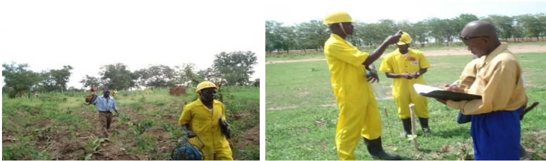
Figure 4-7: Example of Pipeline inspection using a full walking survey method; line measurement, records, and notes are all collated.
