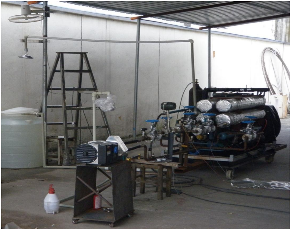
Figure 3-7: LH cogen system: side view 2
