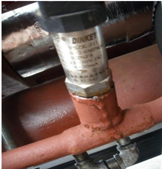
Figure 3-27: Pressure sensor at Evaporator 2
