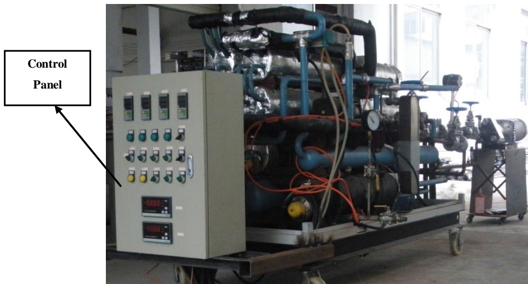
Figure 3-6: LH cogen system: side view 1
