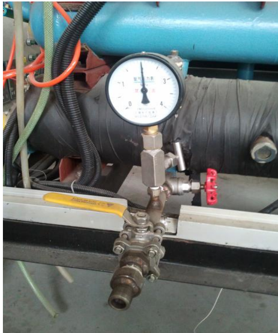
Figure 3-33: Pressure gage at the evaporator
