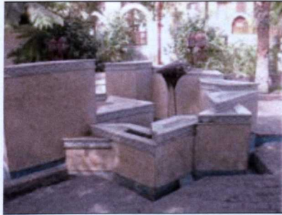
Fig 6.27 Sharp edges and finishing material unsuitable for children
