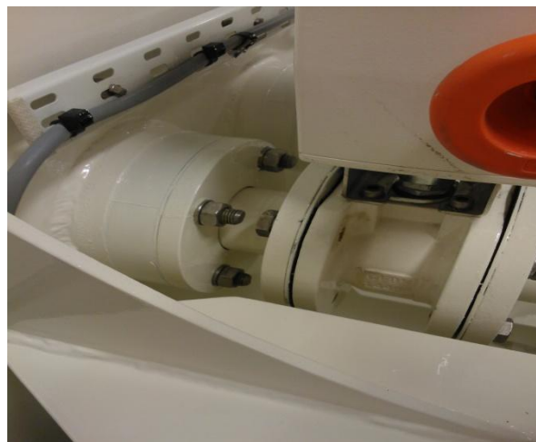
Figure 5-18 Un-coated ballast valve nuts and bolts
