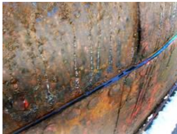
Figure 2-4 Example of uniform corrosion
