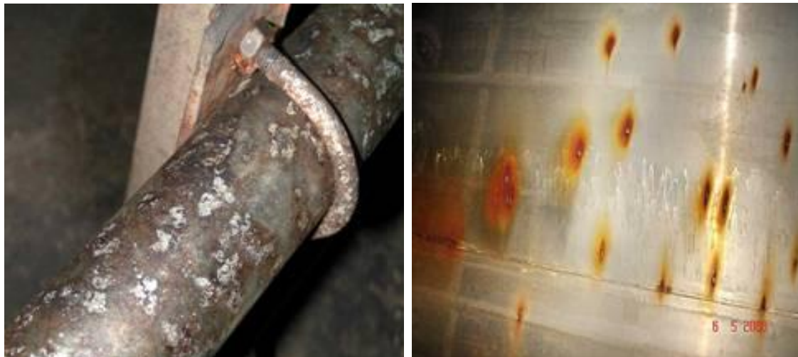
Figure 2-6 Examples of pitting corrosion
