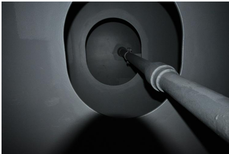
Figure 5-21 Bilge line passing through man hole
