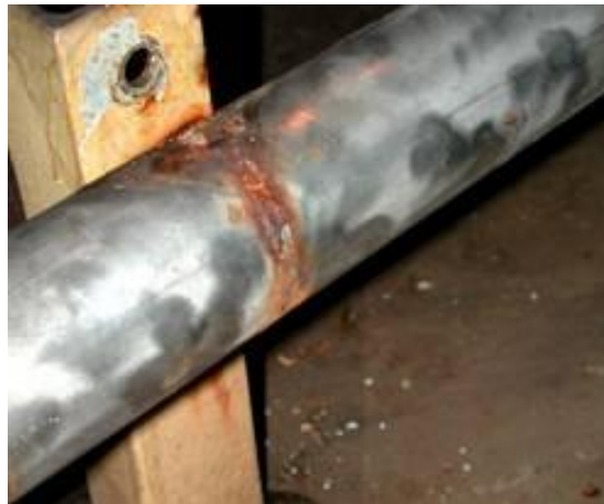
Figure 2-5 Example of crevice corrosion
