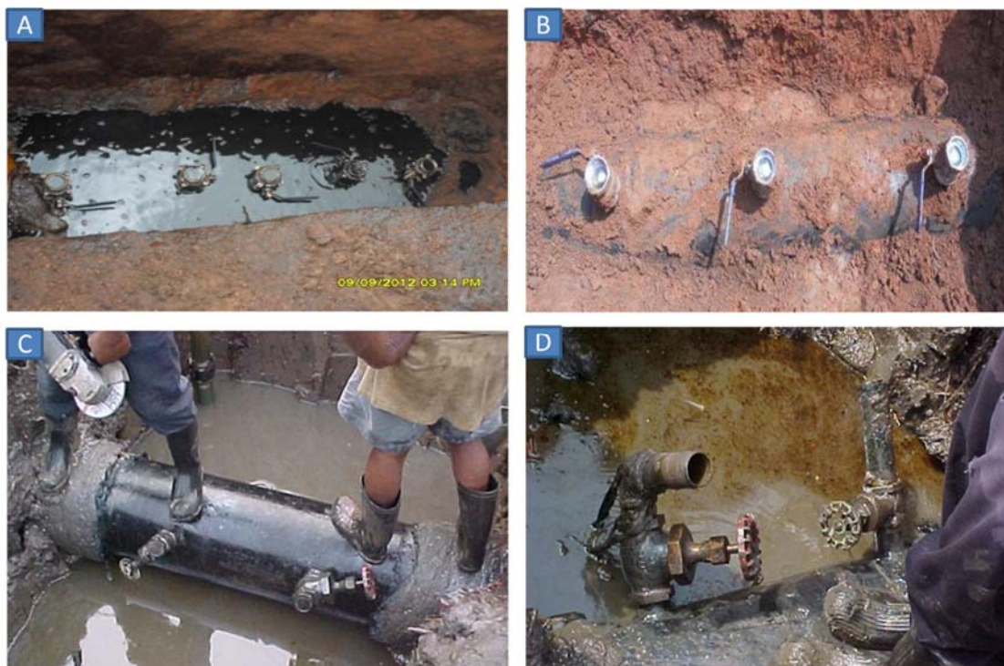
Figure 4-9. Showing unauthorised inserted valves into pipeline (Photo credit A-NOSDRA; B, C and D-PPMC)
