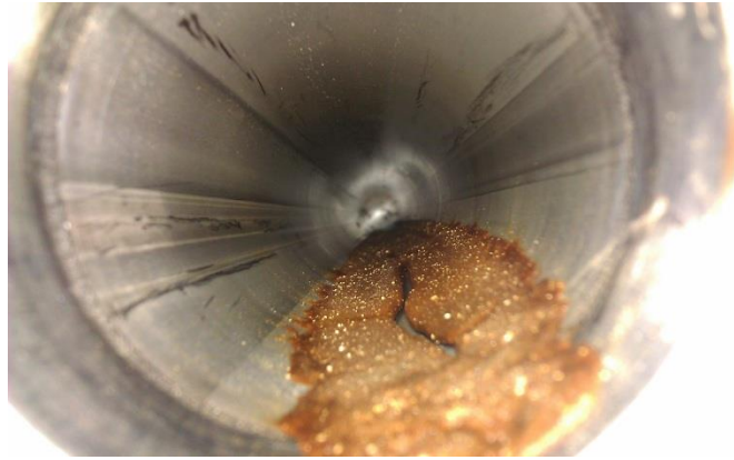
Figure 53: 2 inch Diameter Pipe with Thick Deposit Trail Remaining after Clean
