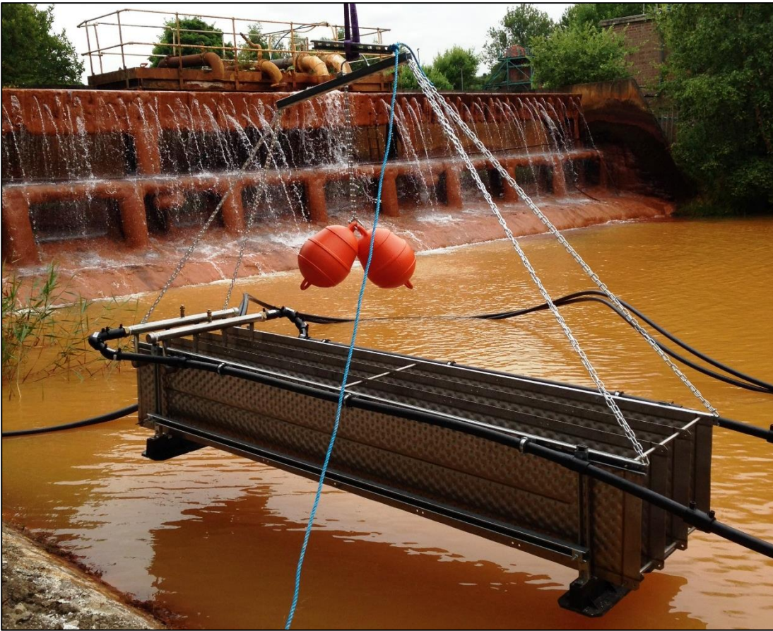
Figure 2.10 Installation of a 'blade' type heat exchanger at Caphouse coal mine water treatment system, Yorkshire, UK (photograph courtesy of Prof. Paul Younger). Note black lines which circulate glycol heat carrier to and from a heat pump.
