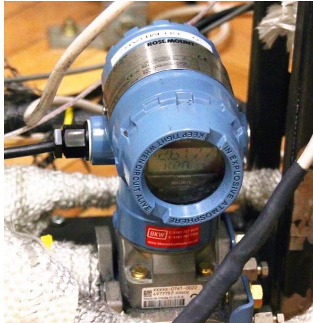
Figure 4-6 Picture of the differential pressure transmitter
