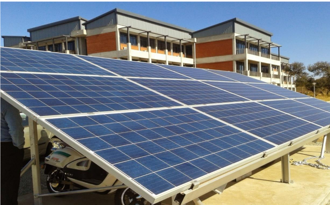
Figure 2.21: Polycrystalline PV modules (Photo taken by the author)
