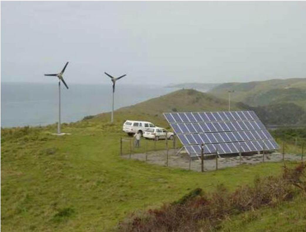
Figure E.1: The wind generator and PV panels in Hluleka hybrid energy system
