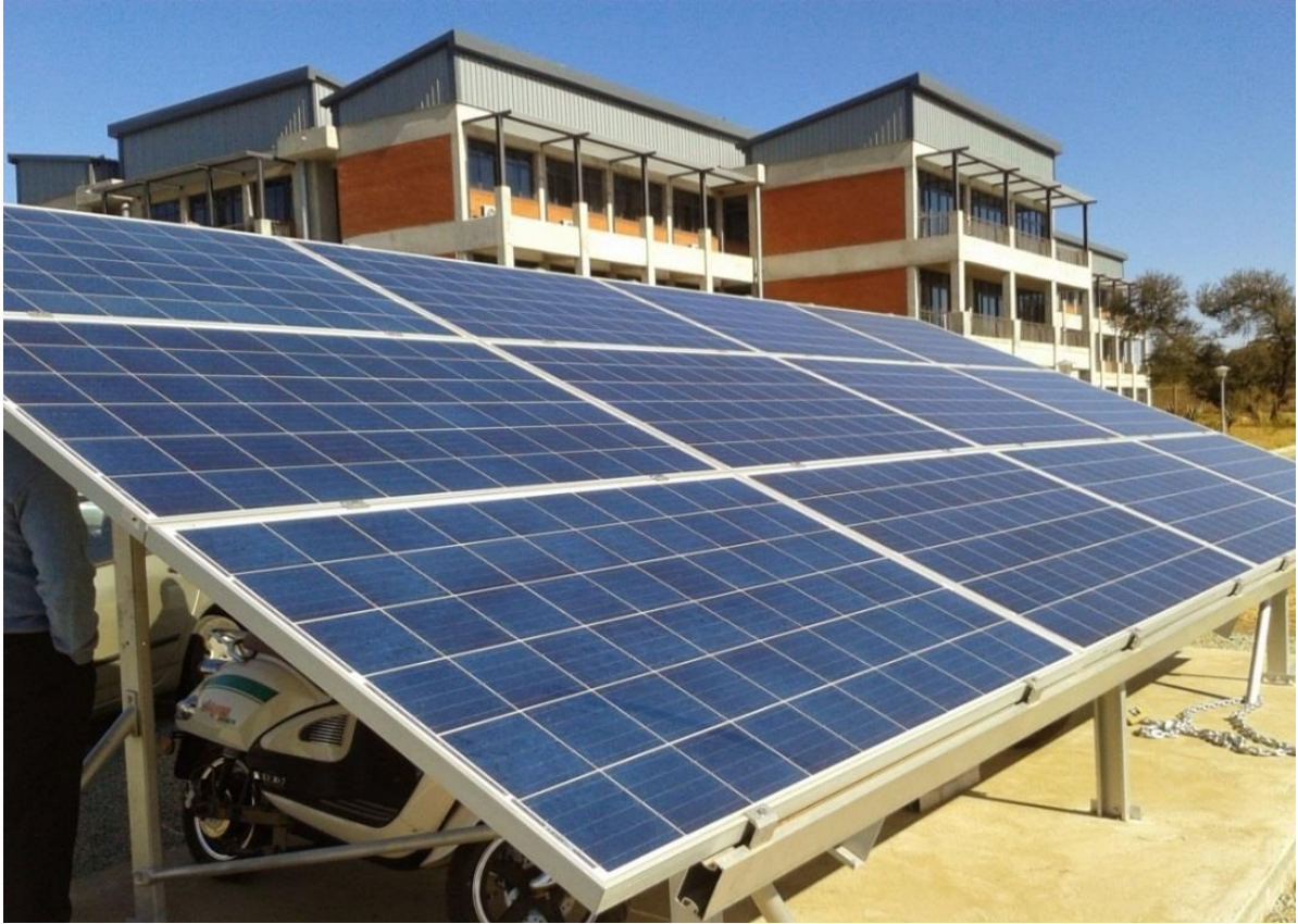
Figure 1.2: Solar PV panels mounted on a roof-top in North West University, Potchefstroom (Photo taken by the author on 31 July 2014)
