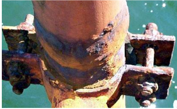
Figure 2.2: Crevice pipe at saddle clamp [21]
