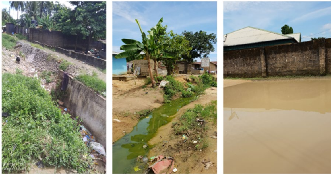
Figure 8.9: The condition of drainage across the study area (especially evident in Mbukpa)
