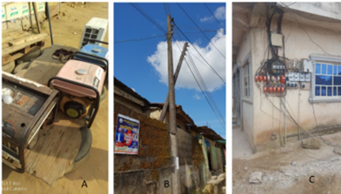
Figure 8.10: A, a generator (used for general and commercial activities); B, illegal electricity connection in Mbukpa; C, pre-paid electricity connection in a multi-occupied house
