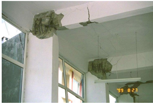
Figure 2.1. After Kocaeli earthquake (1999), damage to RC moment-framed buildings. (Sezen et al. 2003).
