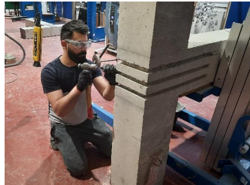
(d) Use a hammer and a hand chisel to remove any remaining concrete lugs and to roughen the surfaces of the grooves.
